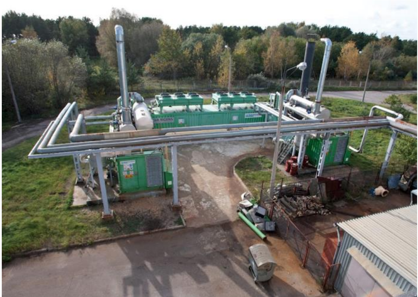
Energy central with CHP, gas flare and heating system in Riga, Latvia. Photo: SIA Rigas Udens.
